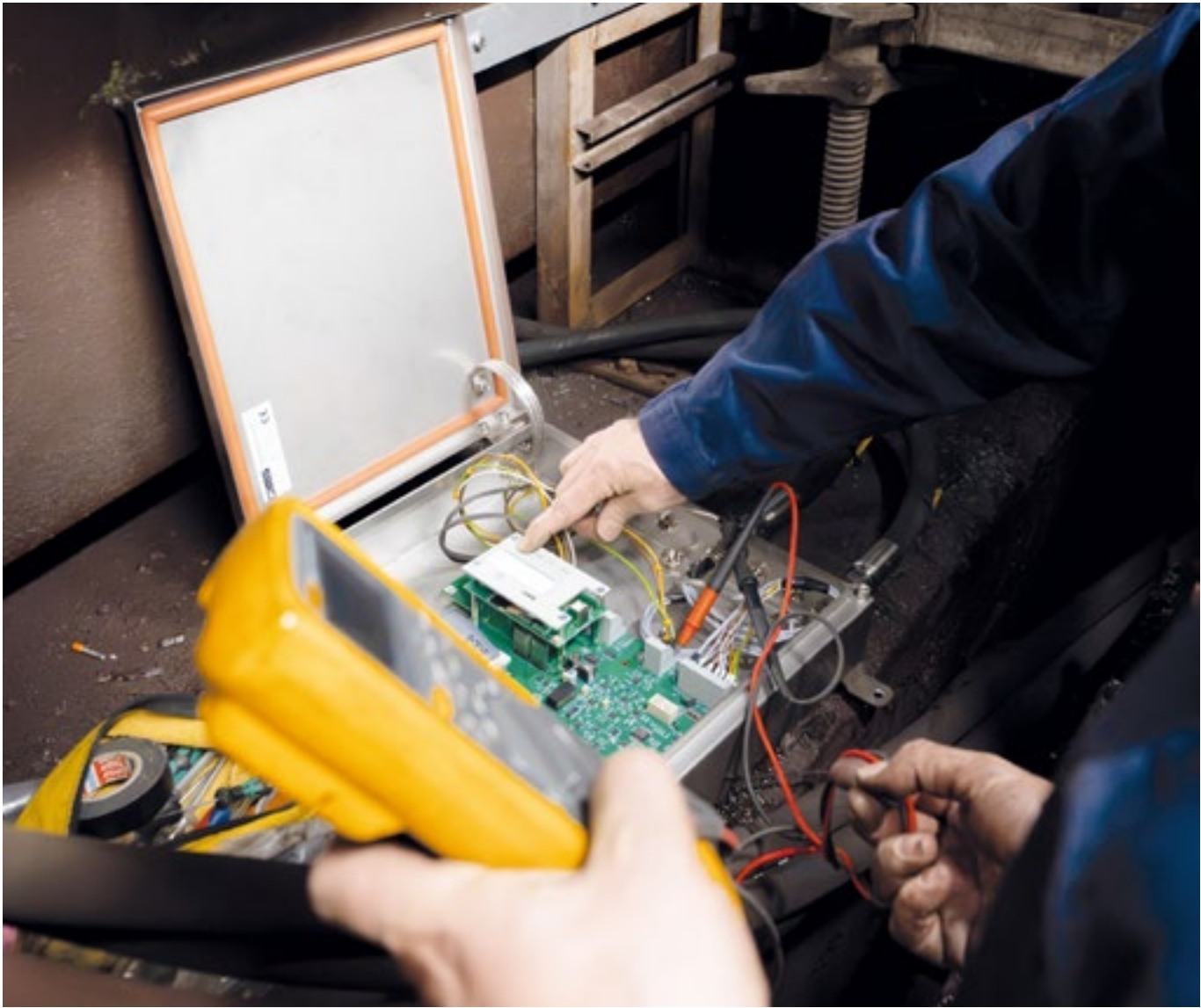
Figure 3: Installation of the StripKraft Controller (MMV) in a hot rolling mill
