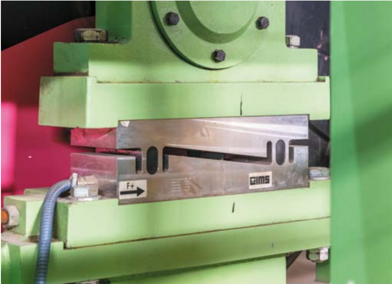
Figure 2: StripKraft HMK in use in a processing line
